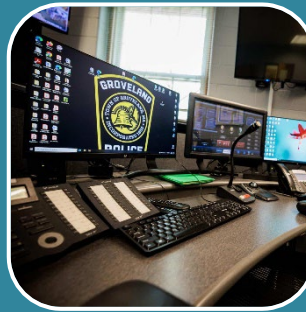
Emergency Communication Systems
