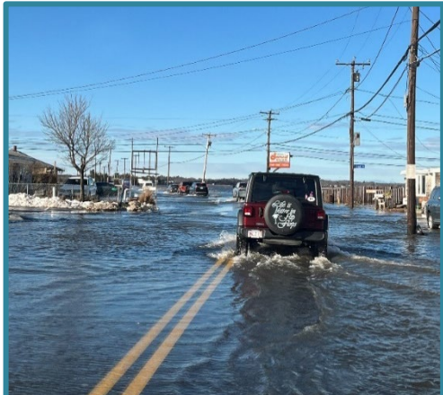
Coastal Flooding Plum Island Tpke, Newbury
