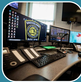
Emergency Communication Systems
