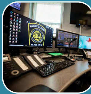
Emergency Communication Systems
