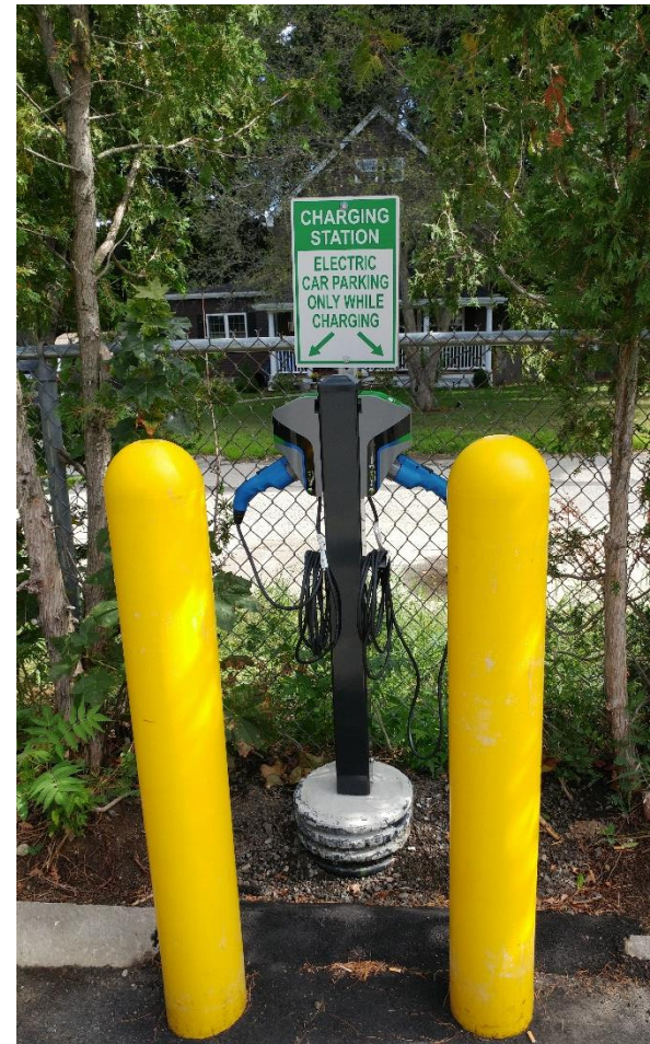
Photo: Chargers for electric cars in North Andover.
