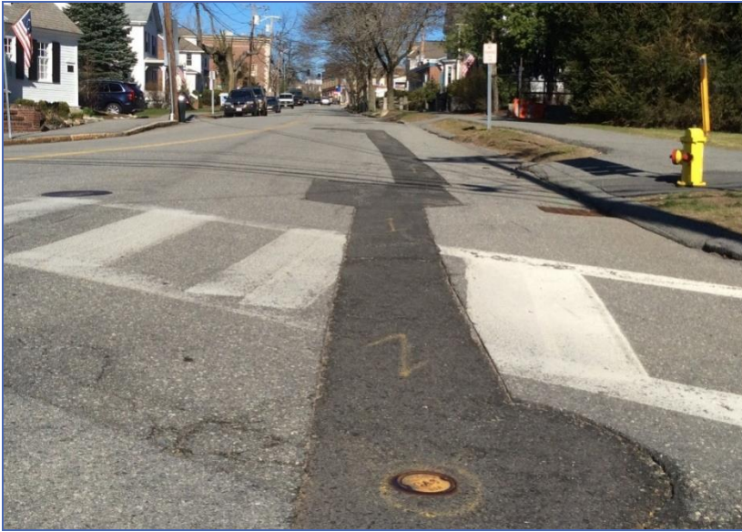
Photo: Section of Chestnut Street in Andover where trenches were dug to repair gas utility lines.
