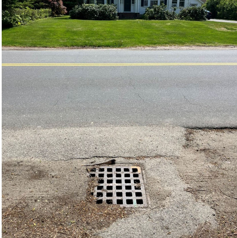
Figure 55. Catch Basin on the Westbound Side of Parker Street near 2 Parker Street
