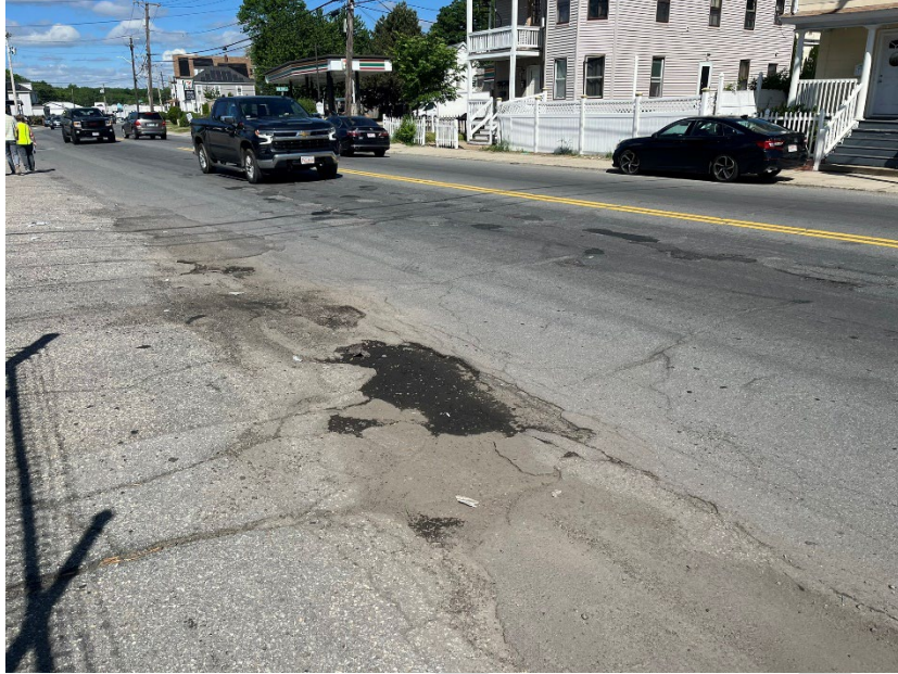
Figure 29. Disintegrating Pavement and No Sidewalk on River Street.
