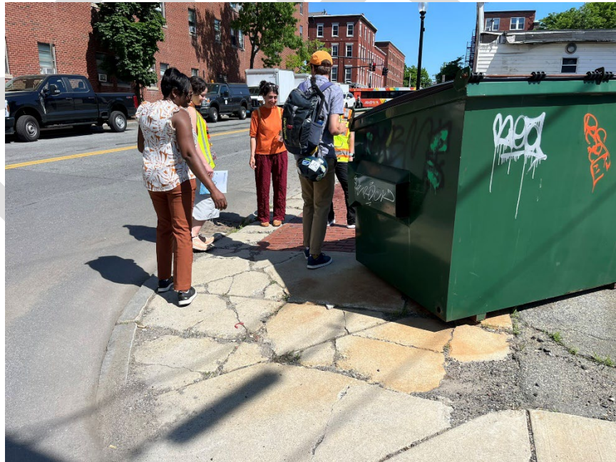
Figure 37. Crumbling ADA Ramp and a Dumpster Blocking the Sidewalk at the Corner of Jackson and Methuen.
