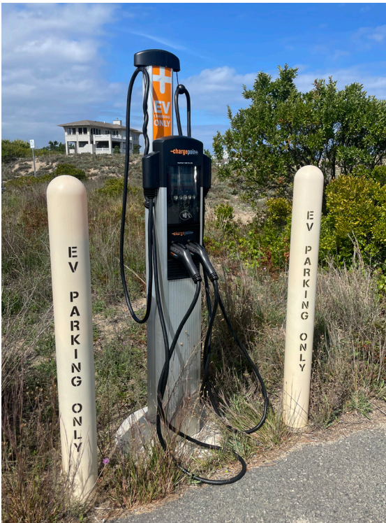
EV Chargers at Parker River National Wildlife Refuge
