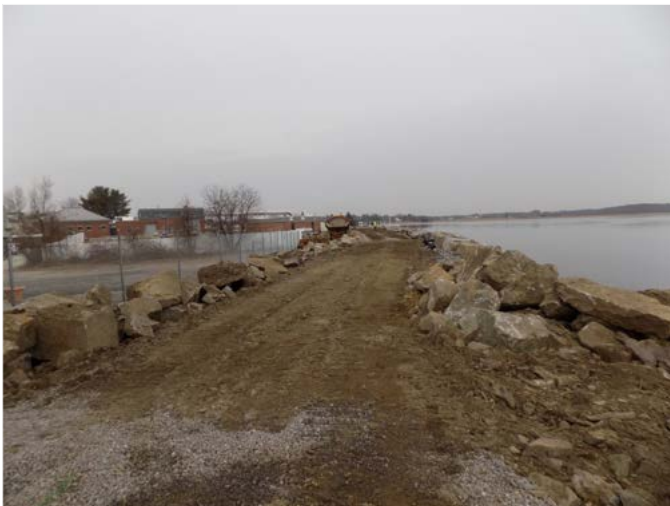
Wastewater Treatment Plant, Newburyport
