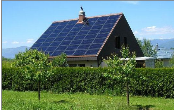
Solar Photovoltaic (PV)
