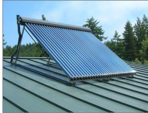
Solar Hot Water
