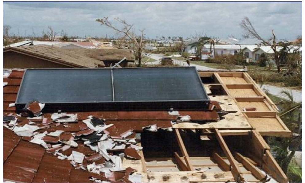
Panels on hurricane damaged roof in Florida. From One Block off the Grid: http://1bog.org/yes-solar-panels-can-survive-a-hurricane/
