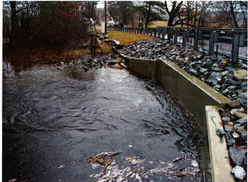
Upstream side of new culverts at East Street during stormwater runoff in March 2010
