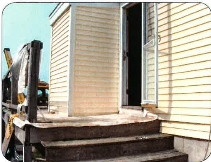
This small addition, built with FEMA assistance, holds a Quincy home's utilities and appliances above projected floodwaters. Thanks to innovative braces, the addition doesn't increase the building's footprint.
