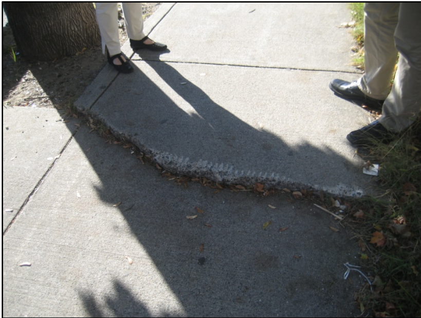
Photo: A walking audit of Winter Street found sidewalks in need of repair. Crumbling sidewalks can be hazardous to elderly and extremely challenging for people in wheelchairs (Photo courtesy of WalkBoston).
