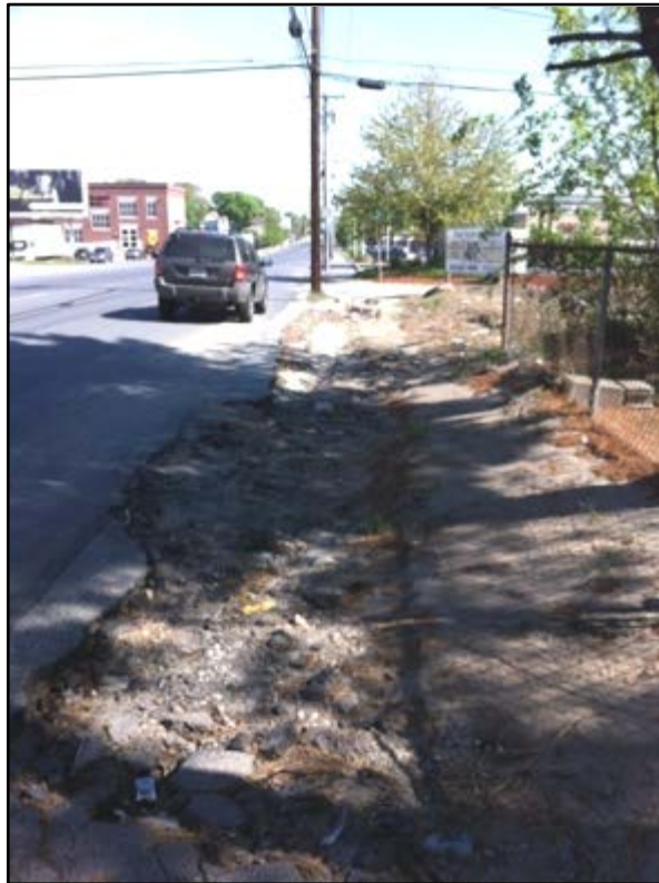
Photo: Significant deterioration of a sidewalk area in Lawrence.
