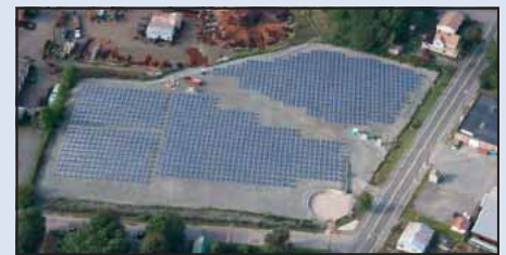
Brockton Brightfield consists of 1,395 SCHOTT Solar modules manufactured in Billerica, MA.
